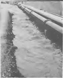
WATER FALLS over a wall in the tank farm presents a unique and rather unexpected sight in an oil refinery. The heavy rain, Nov. 12 caused the falls in the reboiler stream that caused the overflow.
